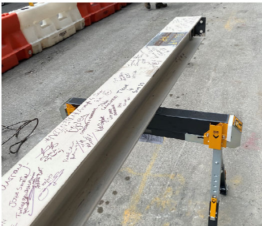
Garden Towers_Final Beam: Project partners signed the final steel beam for Garden Towers before it was lifted into place during the project's recent topping out.
